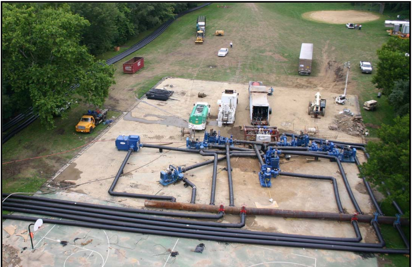
Aerial views of the large bypass project show the size and scope of the application.
