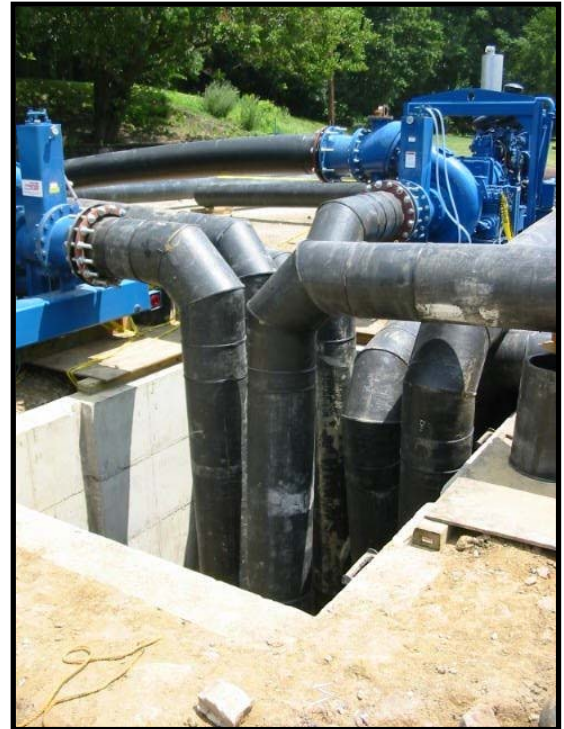
The suction lines of the pumps were inserted into the suction pit to begin the bypass.
