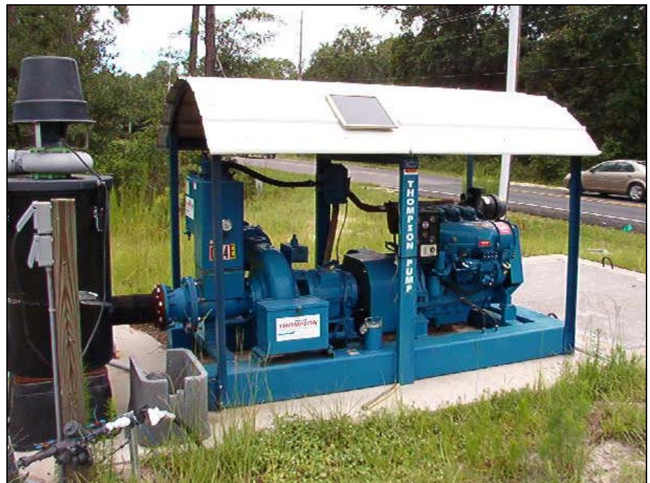
One of ten permanent Thompson Pump emergency back-up pumps used by Regional Utilities in Walton County, Florida. The pumps are equipped with automatic start/stop systems.
