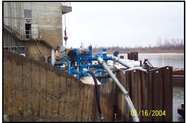
Thompson pumps dewatering the coffer dam to allow crews to make repairs to the Johnson County Water Treatment Plant.
