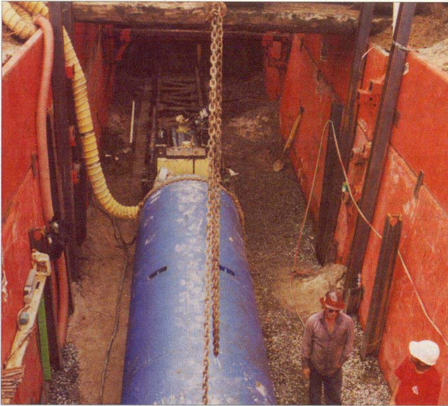
Atlanta Boring & Tunneling crews prepare to launch a drive of 54-in. casing for Macon (Ga.) Water Authority.
