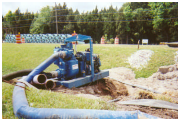
Thompson Pump's 6-inch Dry Prime Pump with SuperSuction Vacuum-Assisted Priming System dewateres a water line.
