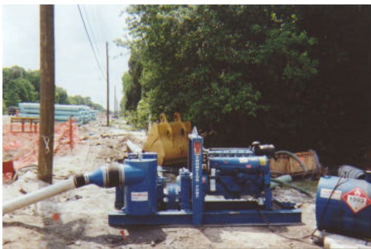
An 8-inch Thompson Rotary Wellpoint Pump on the Nova Road project with external fuel tank for extra fuel capacity.
