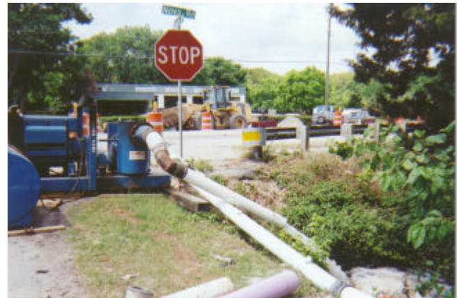
A Thompson 12-inch Rotary Wellpoint Pump using a wellpoint system temporarily lowers the water table enabling crews to excavate without the worry of the presence of water.
