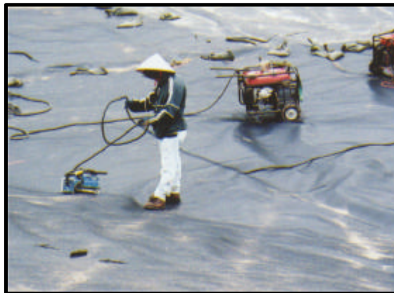
Above Right: Liner is placed on the bank of one of the lakes.
