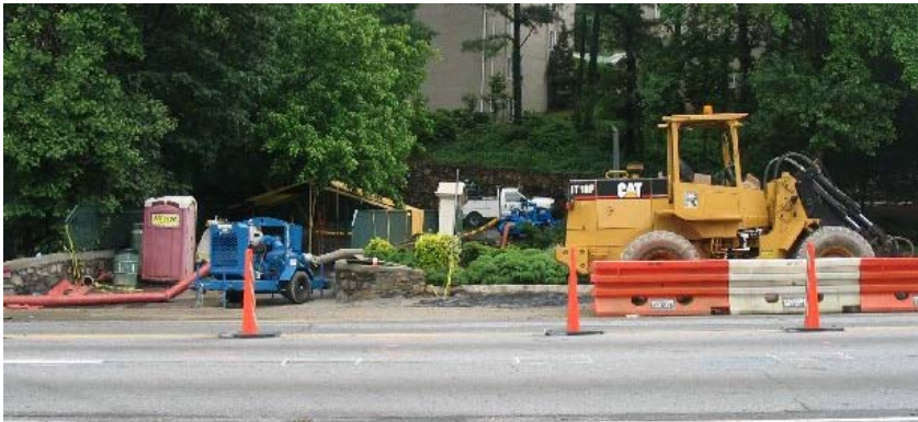
The quick response by Thompson Pump allowed GDOT crews to begin repairs to Roswell Road and the retention wall bringing traffic back up-to-speed.
