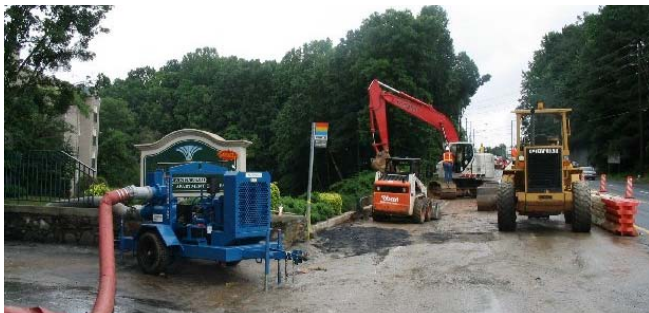
GDOT crews repair Roswell Road while a Thompson Pump 8-inch Dry Prime Compressor-Assisted Trash Pump dewatering the four acre lake.
