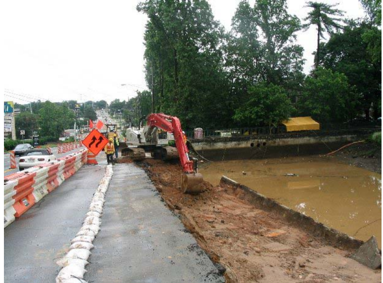
Heavy rains caused Roswell Road to crack and collapse causing the retention wall along the lake to collapse as well, causing flooding on the heavily traveled northbound lanes.
