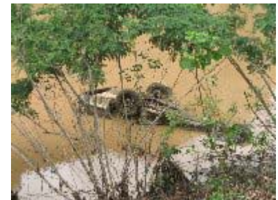
A trailer that fell into the retention pond when Roswell Road collapsed.
