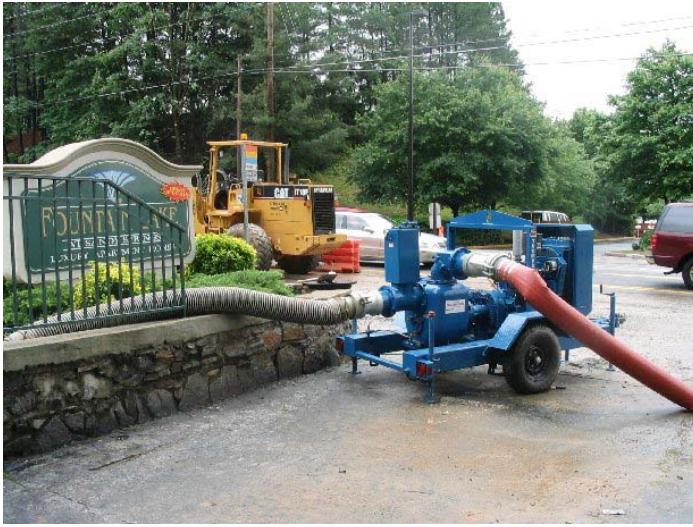
Thompson Pump's 8-inch Dry Prime Compressor-Assisted Trash Pump reduces the flooding threatening Fountain Lake Apartments
