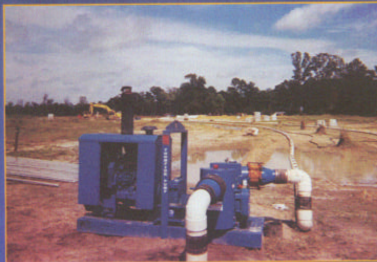
Figure 1. Thompson's 6-inch vacuum-assisted pump is used to drain water from trenches so excavation can continue.
