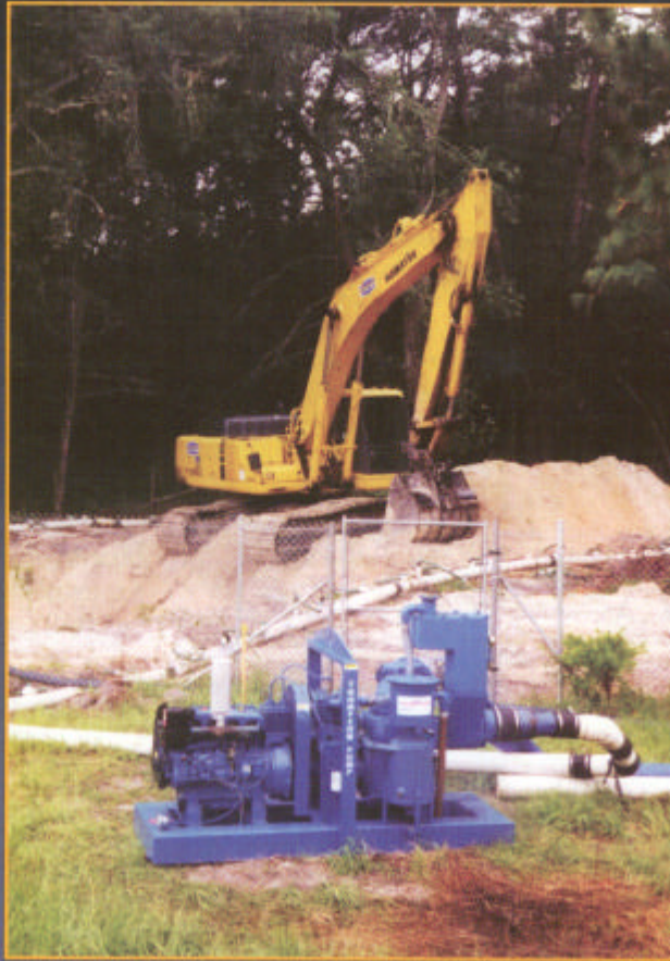
Figure 2. Large areas of land can be dewatered with a Thompson wellpoint system.
